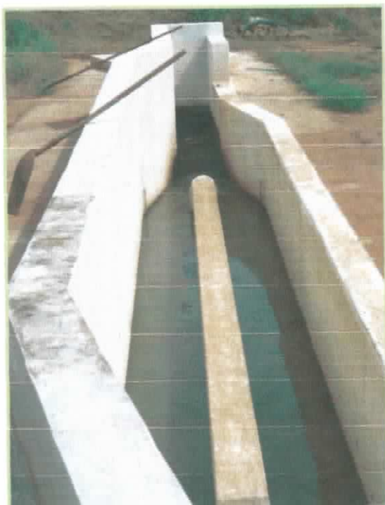
Foto 21 - Canal com as grades
