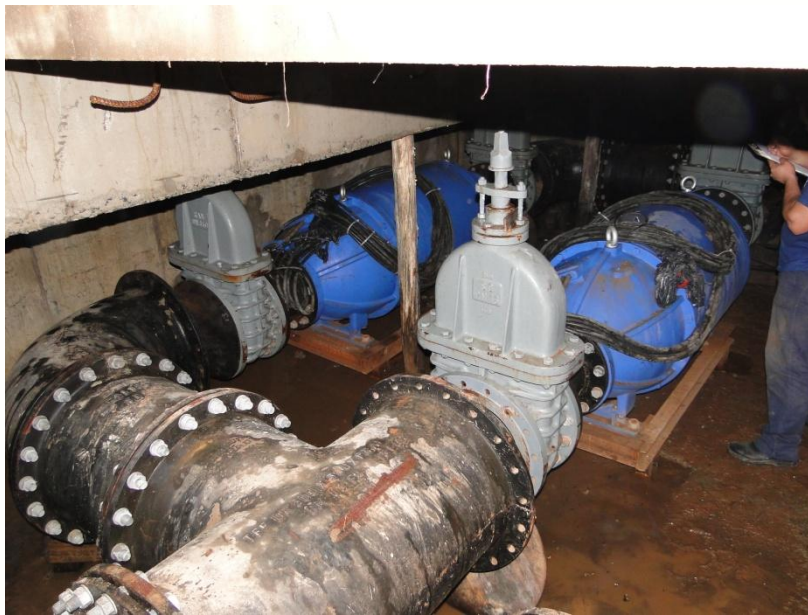
Figura 87 – Bombas do booster San Martins.
